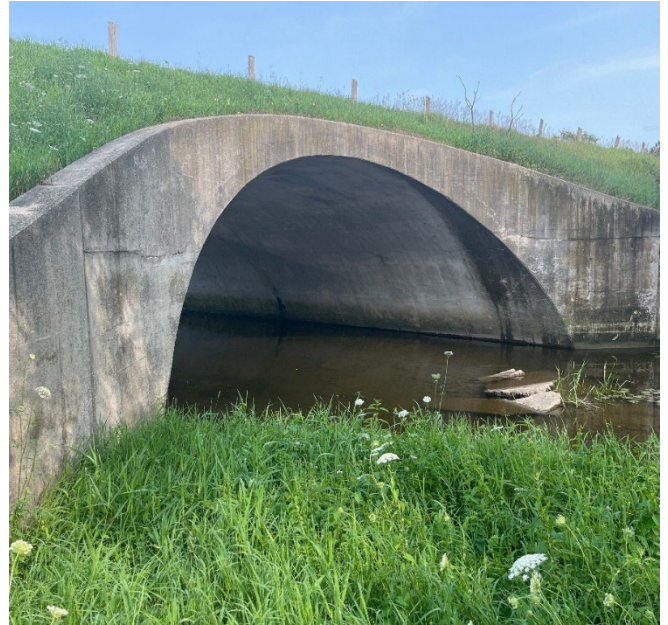
Figure 3.1-1 Example of a County CSP arch OSIM culvert (C060800, Wellington Road 6, Minto).
