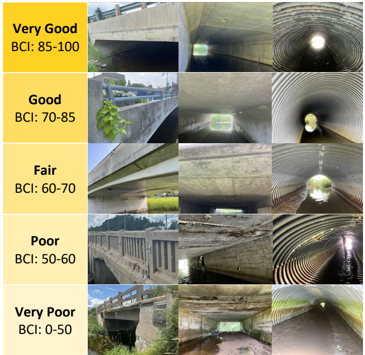
Figure 3.1-6 These images of County bridges and structures reflect the different condition ranges.
