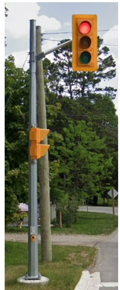
Figure 3.5-2 Example of a County traffic signal (WC-TS-041) along Wellington Road 18.
