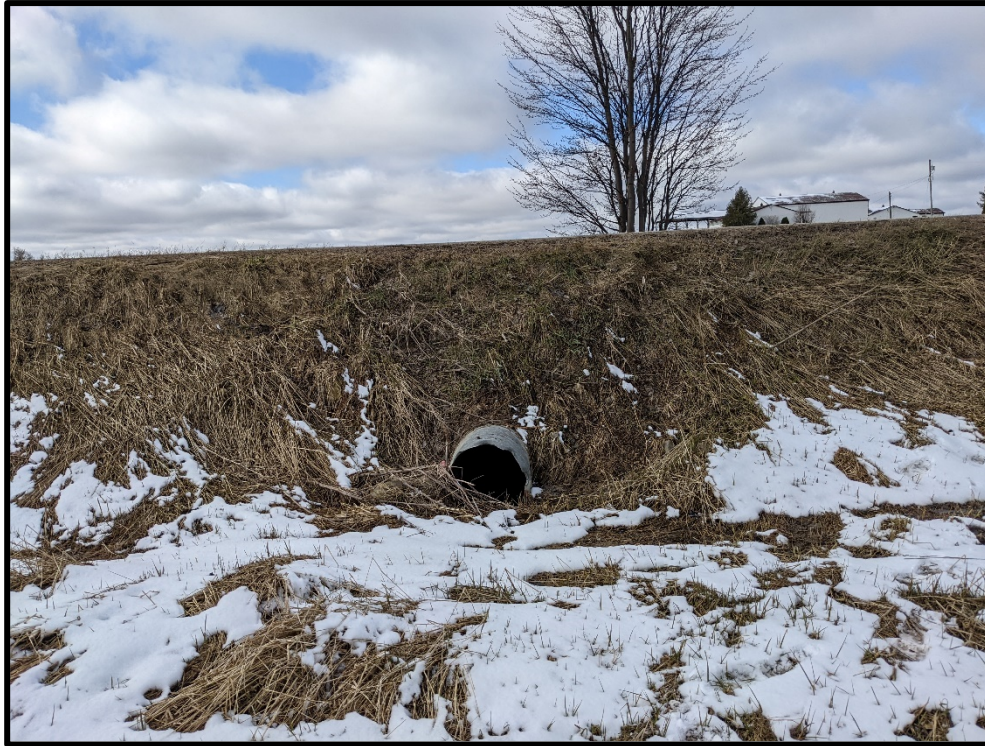
Outlet of low-lying wetland area, 600mm diameter CSP culvert crossing King Street
