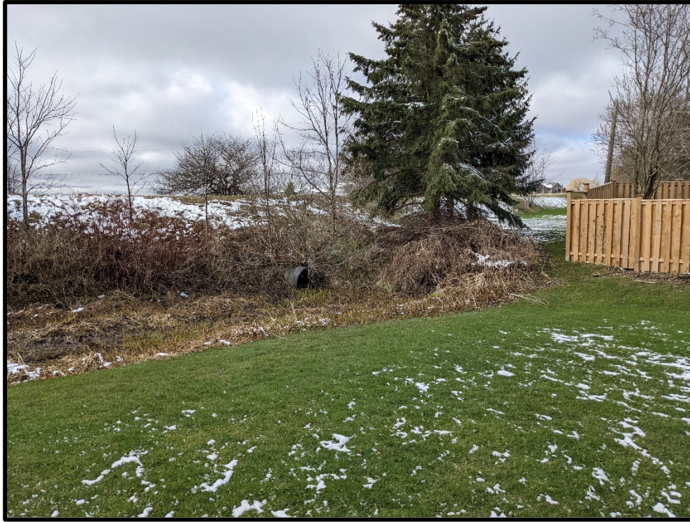
900mm x 770mm CSP culvert crossing rail trail at vacant lot on Bell Street
