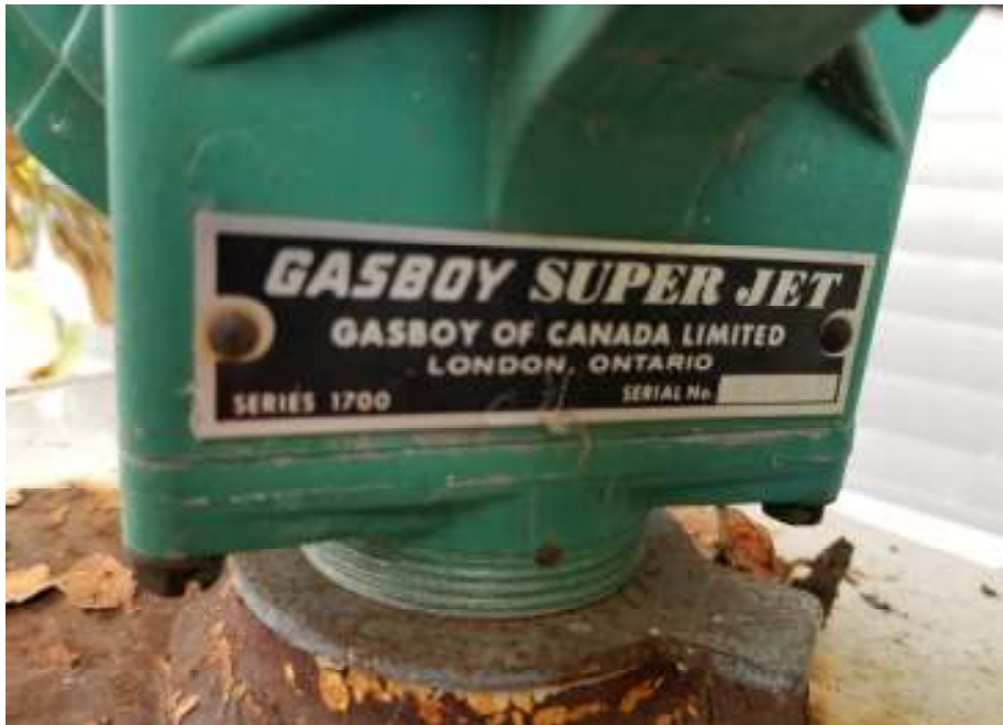
Photo 5 - Photo of the tag located on the diesel fuel tank.
