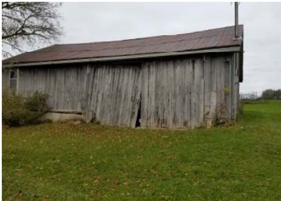
Photo 2 - East view of the existing shed located at the southwest end of South Mill Street.
