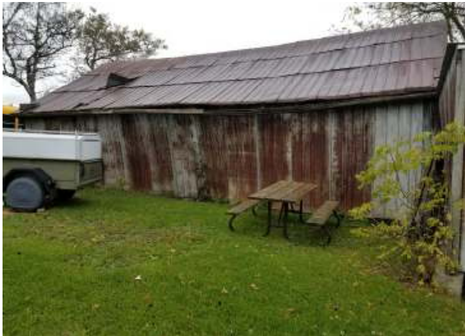
Photo 7 - View of the west face of the existing shed located at the southwest end of South Mill Street.
