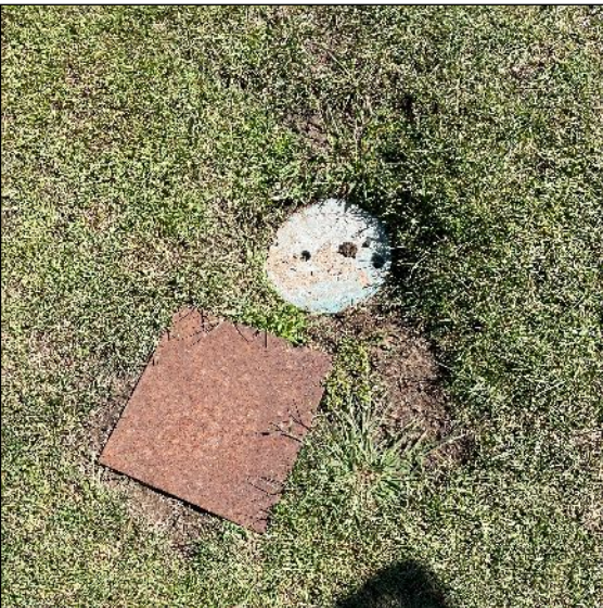
Image 19: Example of in-ground utility.
