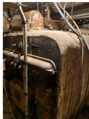
Picture 6: View of electric boiler in the clubhouse basement.
