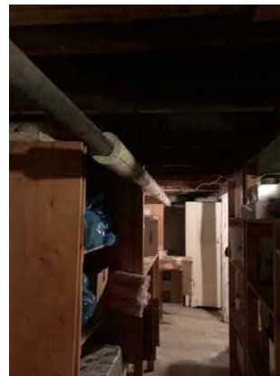
Picture 4: View of the clubhouse basement with potential asbestos containing pipe wrap.
