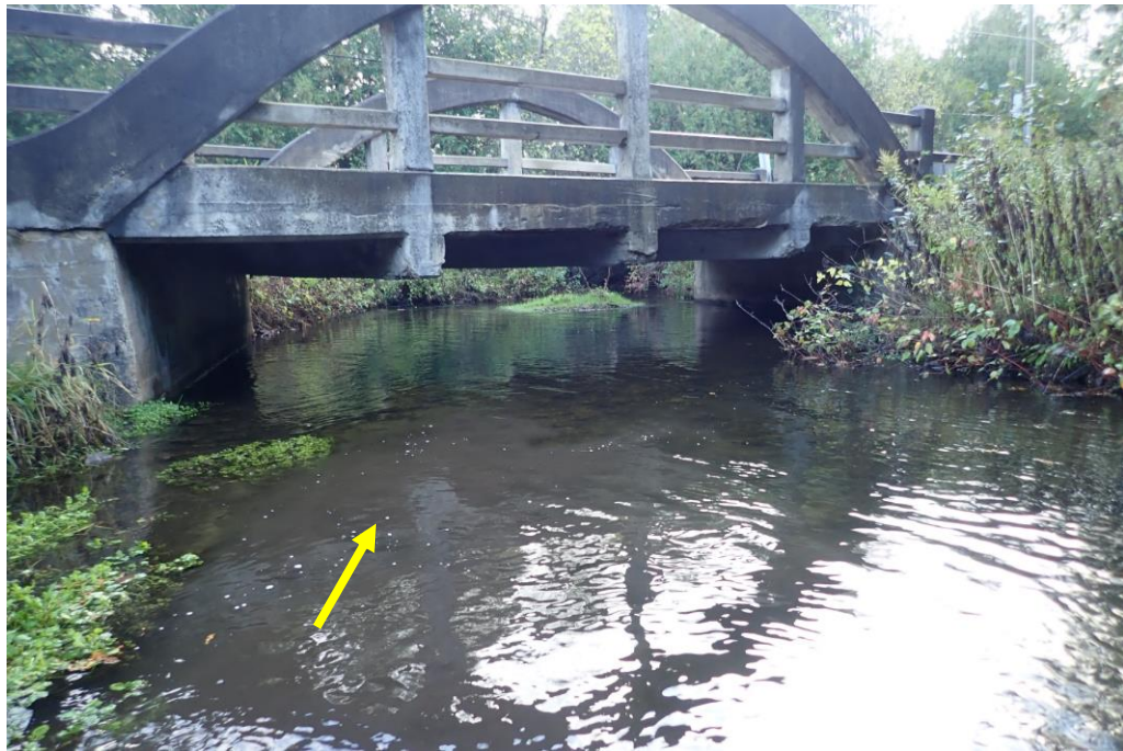
Despite the wetted width of the channel extending to both footings, no significant evidence of instability was observed for the 8 th Line bridge crossing.
