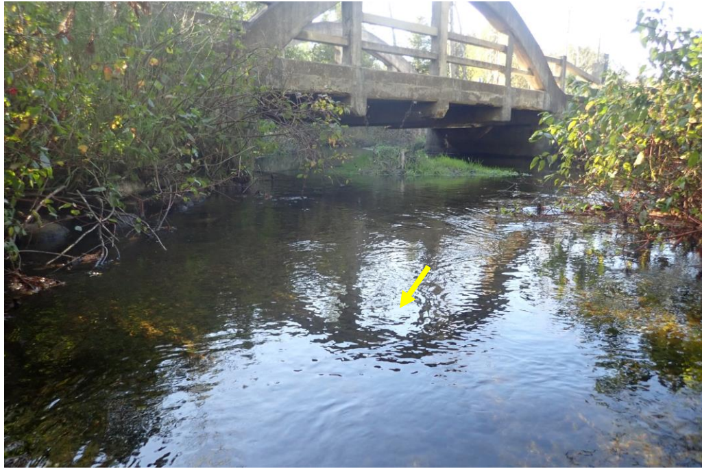
Photo taken facing upstream at the 8 th Line bridge crossing. The yellow arrow denotes flow direction.
