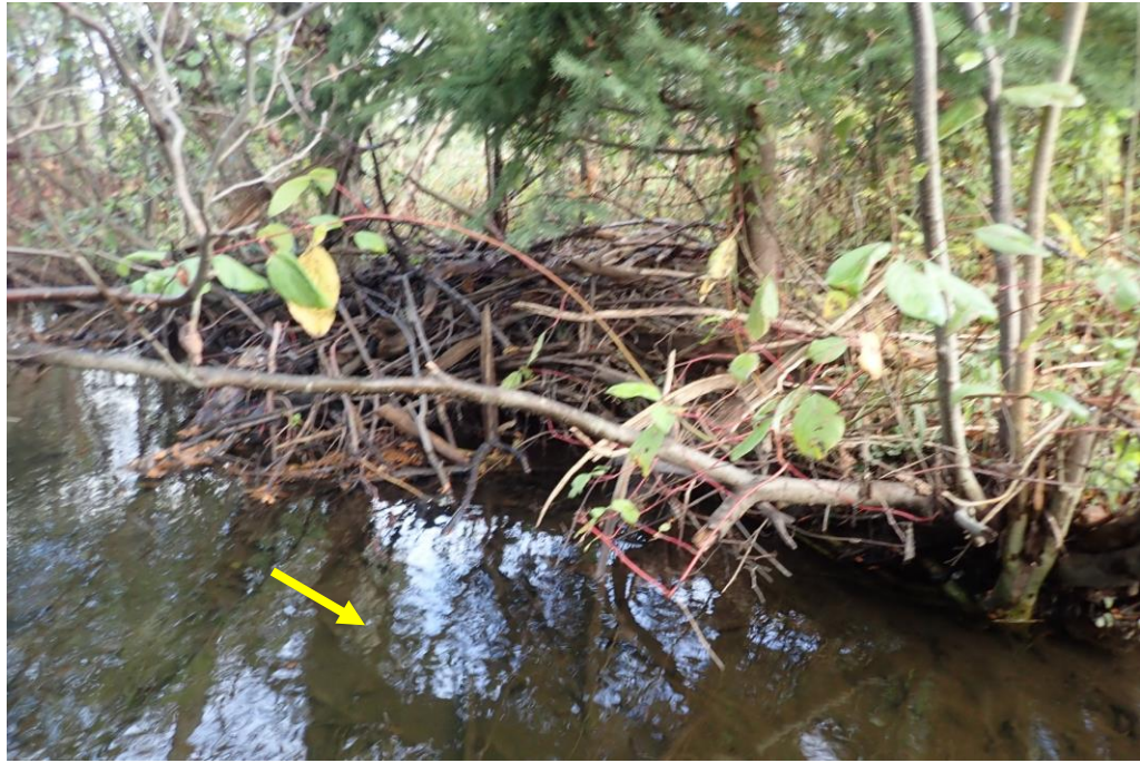
Exposed roots were predominantly from mature trees. Minor bank undercutting was observed in several locations.
