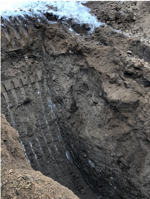
Photograph 2 – View of excavation for TP 102. Test pit was dry upon completion, however, after 4 hours, slow water seepage was observed at 2.5 m below existing grade.
