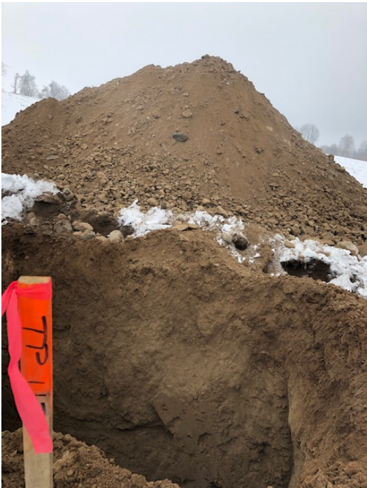
Photograph 16- View of excavated soils from TP 112. After 4.5 hours, test pit was dry and no cave-in observed.
