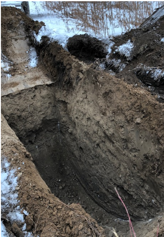
Photograph 8- View of excavation for TP 107. After 4.0 hours, test pit was dry and no cave-in observed.
