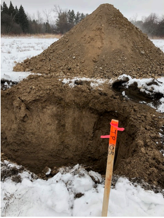
Photograph 5- Excavated soils from TP 105. After 4.0 hours, cave-in of sides and water level were observed at 3.0 m below existing grade.
