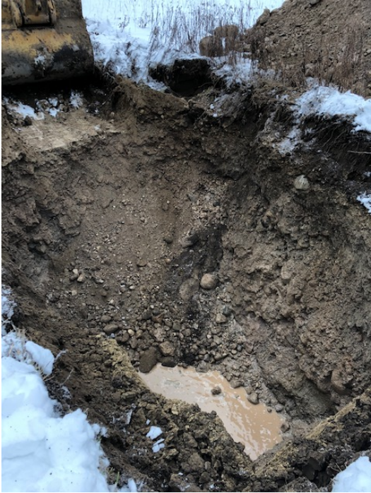
Photograph 7- View of TP 106, note cave-in and water level approximately 0.75 hours after excavation.
