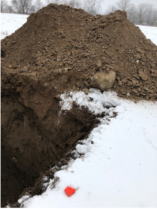
Photograph 1- View of excavated soils for TP 101. Test pit was dry upon completion and no water seepage observed.
