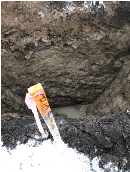
Photograph 10- View of TP 108, approximately 8 hours after completion. Slow water seepage was observed at 2.5 m below the existing grade.
