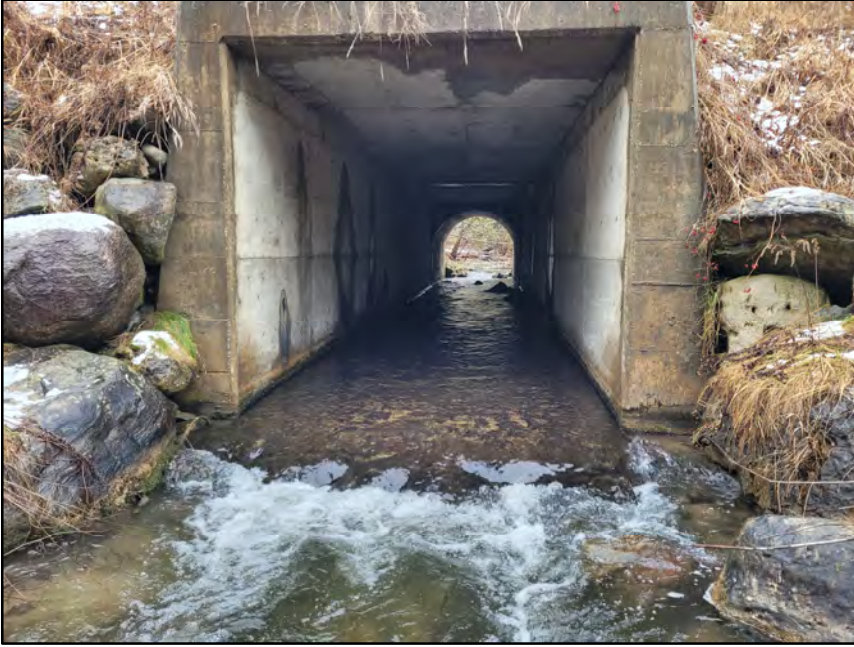
Photo 1. Facing WNW, downstream of Wellington 22. Elevation change creating a minor drop into a plunge pool at downstream extent of culvert.
