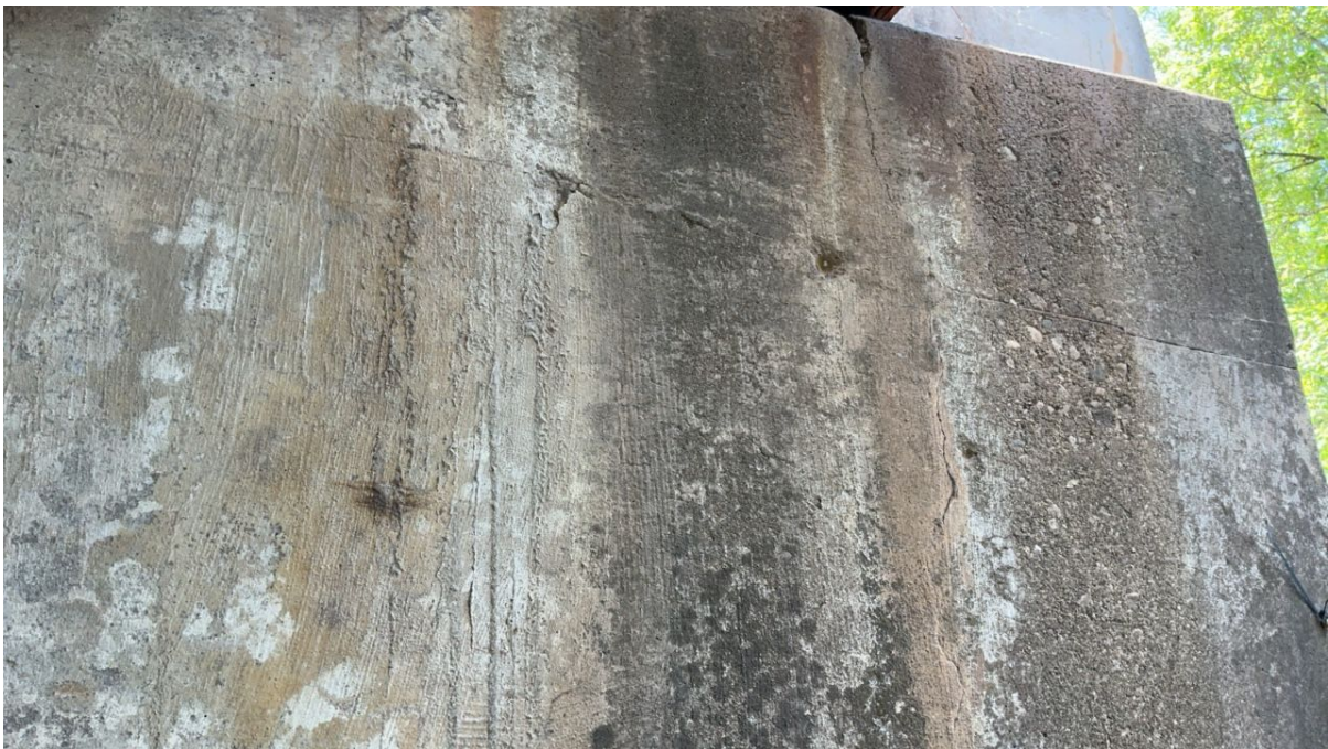
Narrow vertical cracking on South abutment.
