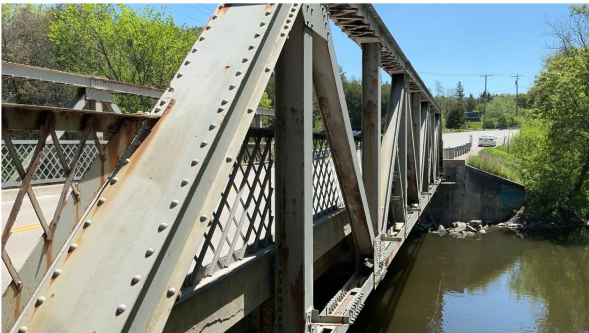
Rust staining on vertical and diagonals (typ).
