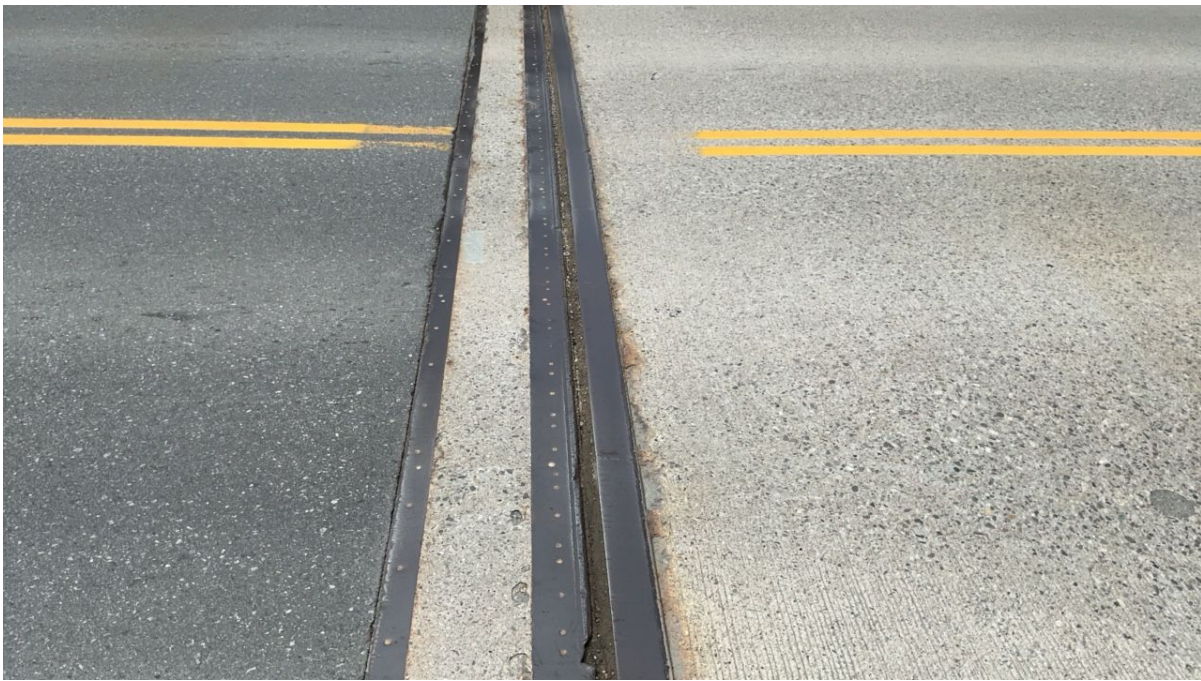
South joint filled with debris.
