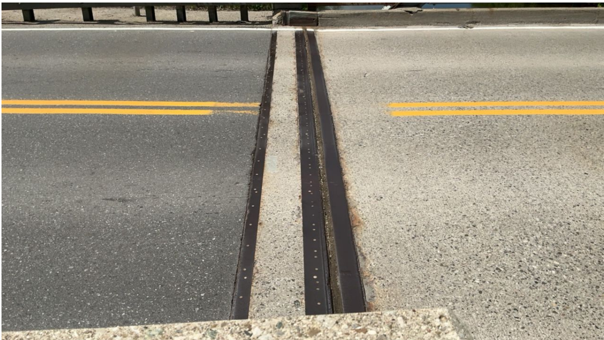
South joint with chip marks from snow plows.
