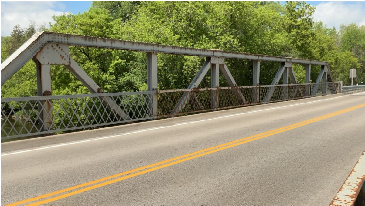
West railing with rust and impact damage.
