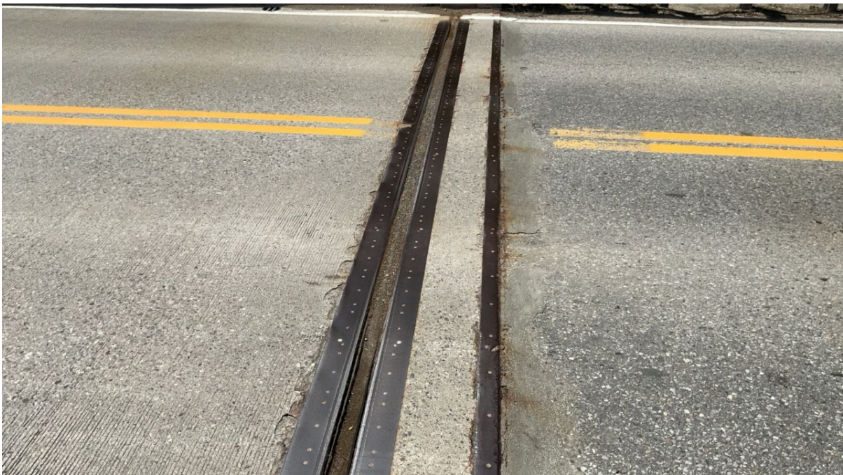
Concrete spalled from North joint.
