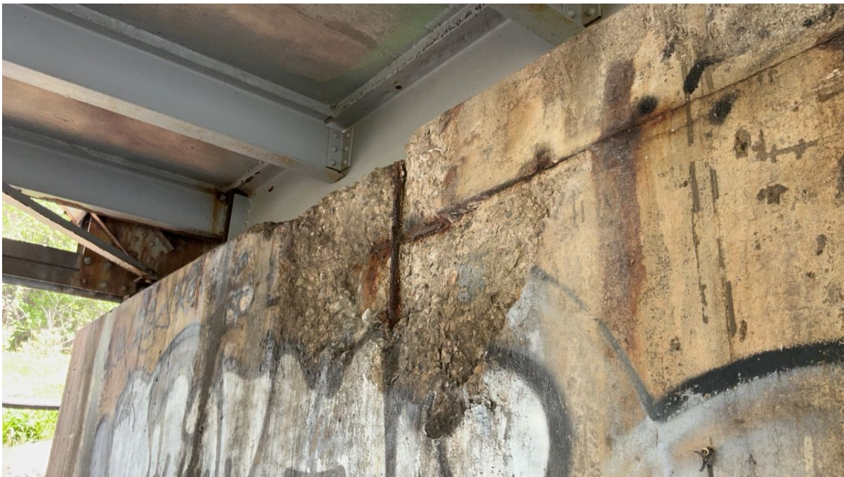
Large spall on South abutment.
