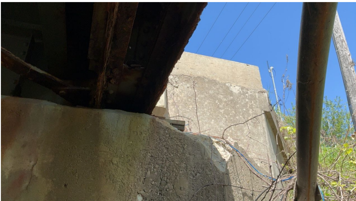
Spall at NE.
