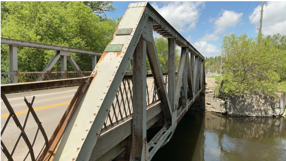
East vertical/ diagonals with rust (typ).
