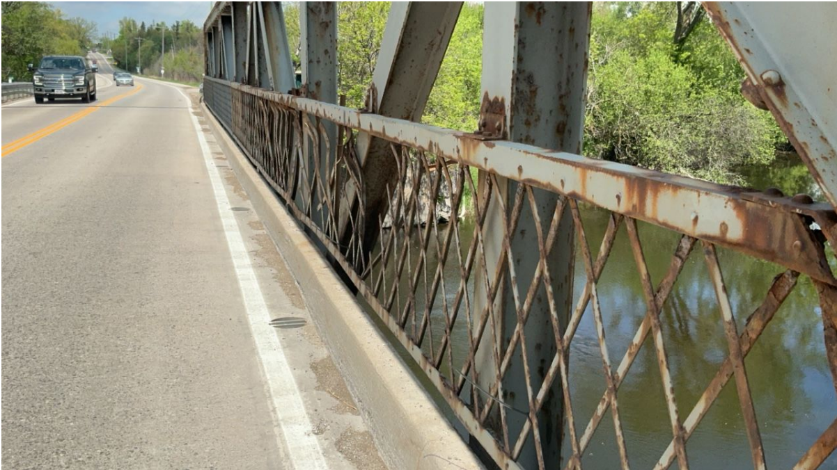
East railing with rust and impact damage.
