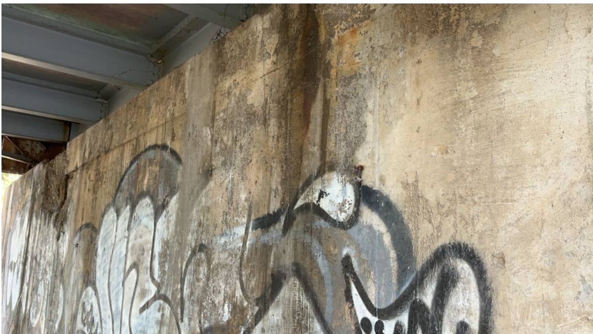
Concrete staining on South abutment.
