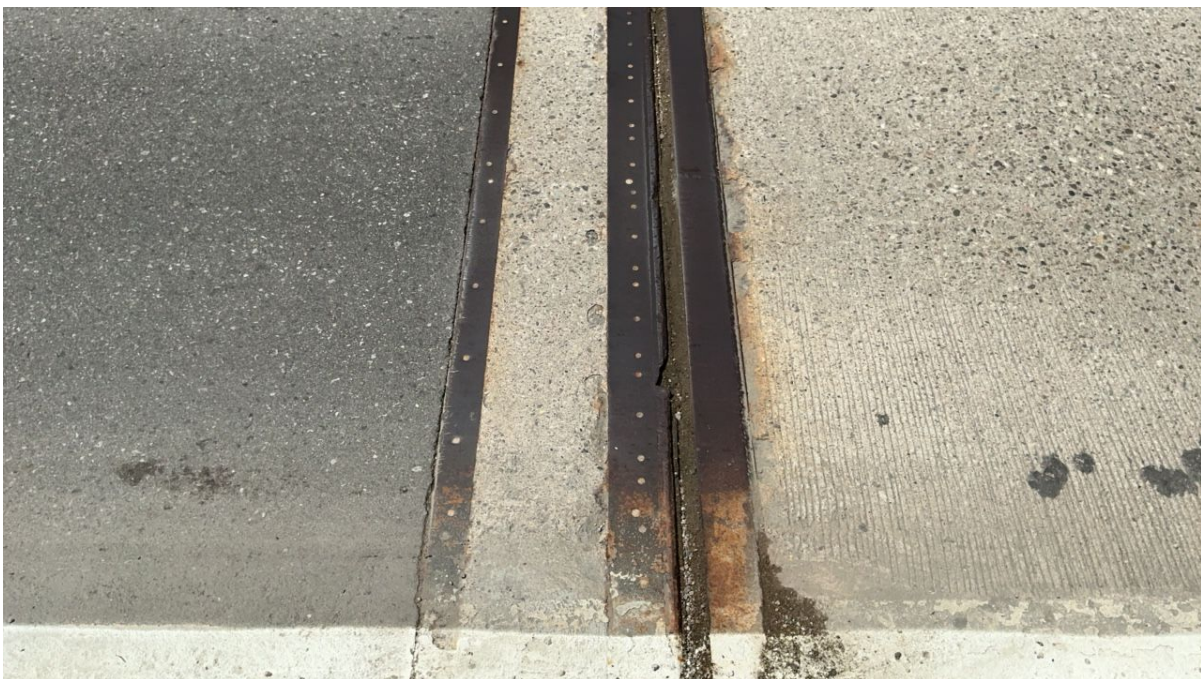
Scaling on South dam.
