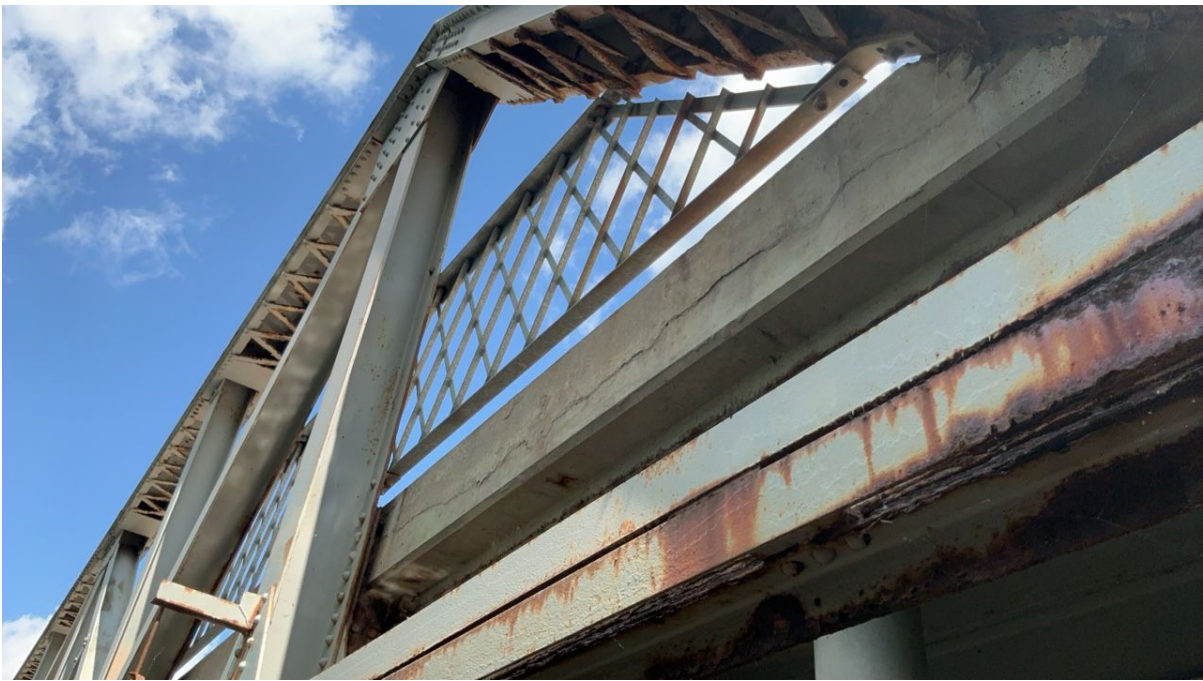
Cold joint on West exterior soffit.
