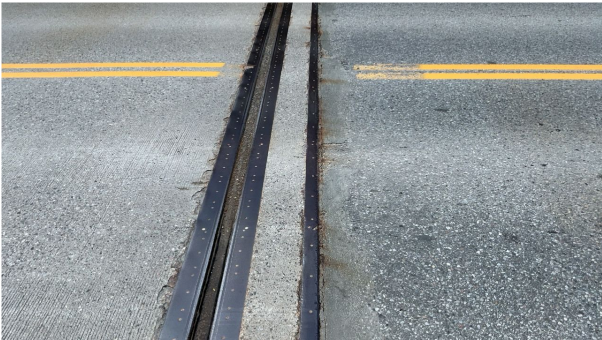
North armour damage.
