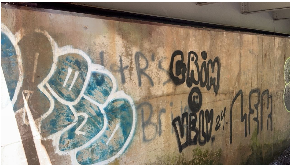
Horizontal crack along North abutment.
