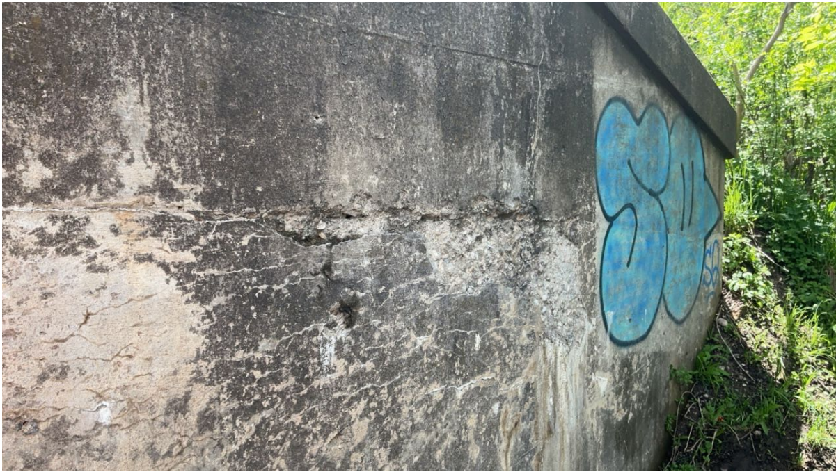
SW wingwall scaling and delamination.
