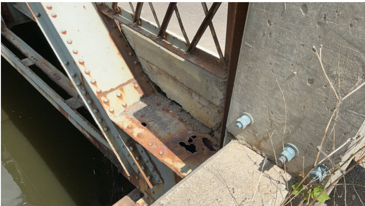
SW end perforation.
