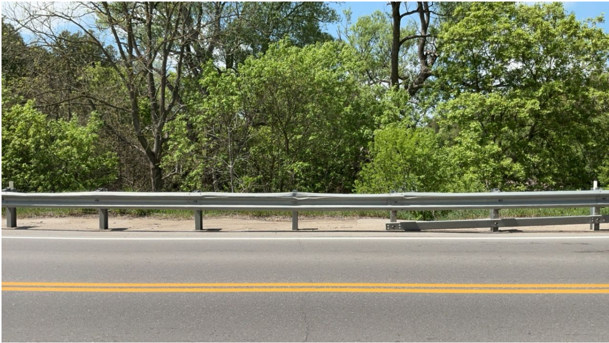
Impact damage on SW guide rail.
