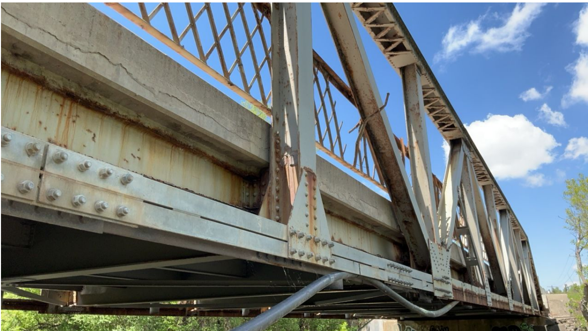
East exterior soffit cold joint.
