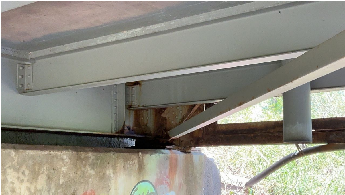
NE bearing with minor spall.
