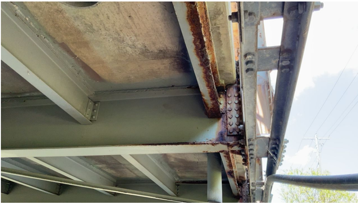
Floor beam rusted connection with bottom and vertical cord (typ).
