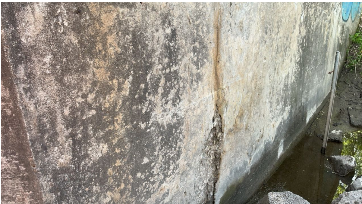
SW wingwall vertical stained cracking.
