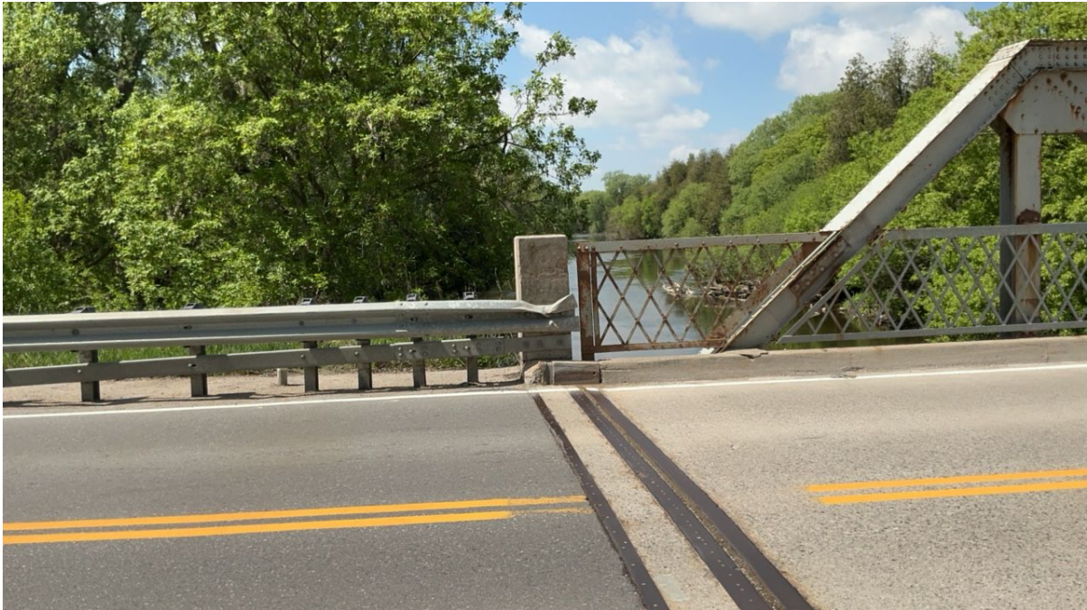
Impact damage at SE guide rail end.
