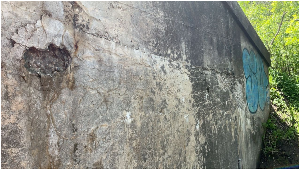
Typical cracking on wingwalls.
