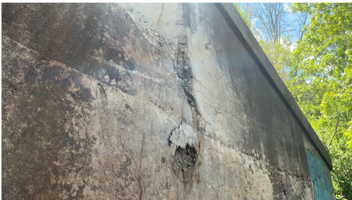
SW wingwall spalls with delamination.
