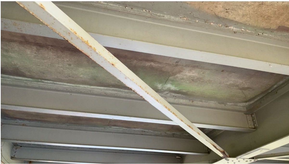
Light bracing rust.
