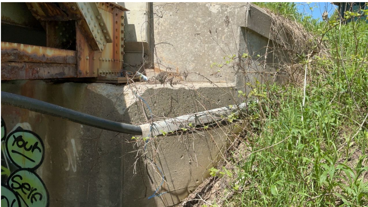
NE wingwall spall and scaling.
