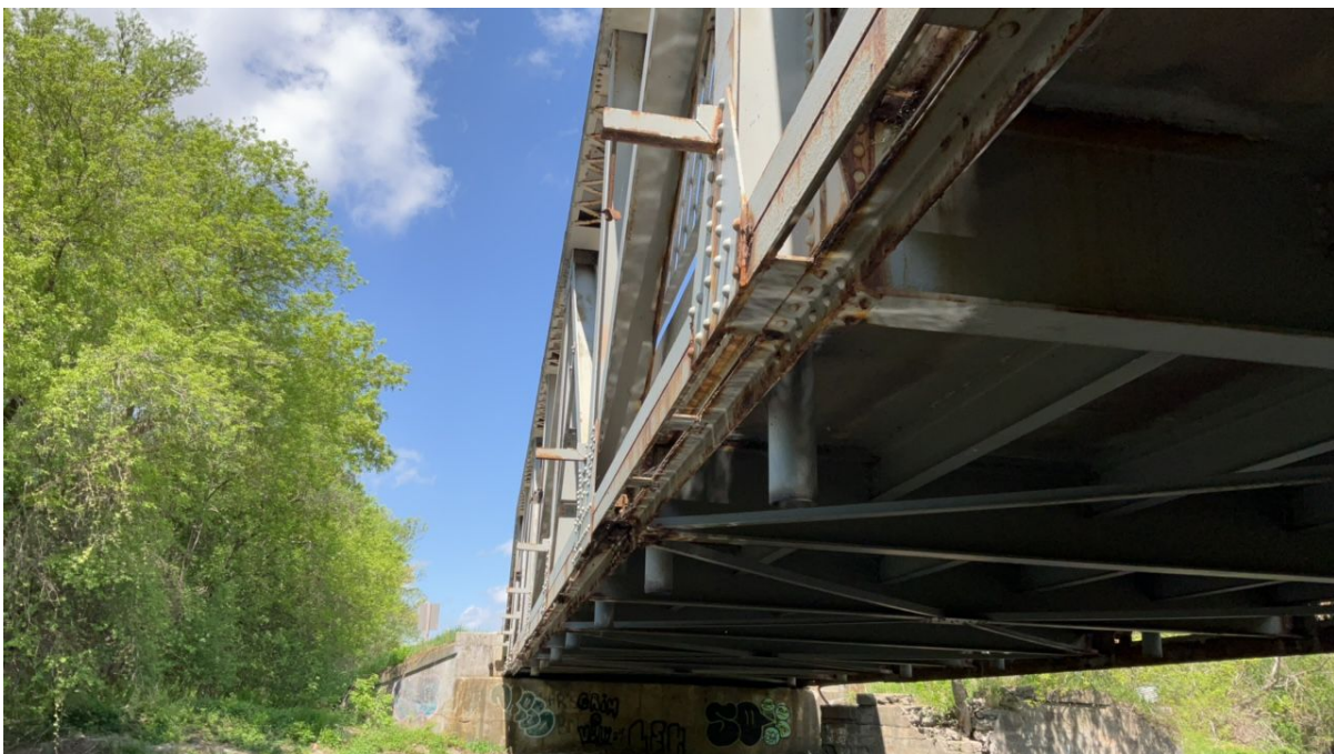
West abandoned utilities.
