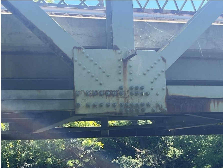
Figure 15: Gusset plate with riveted and bolted connections (A.S.I., 2024).
