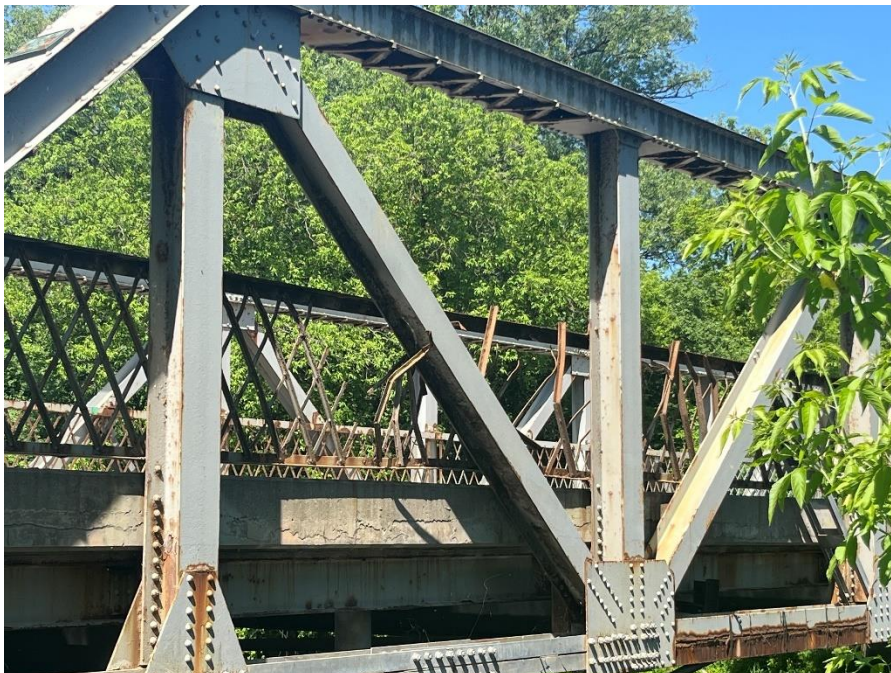
Figure 16: Detail of the vertical and diagonal chords. Note the damage to the lattice railing (A.S.I., 2024).
