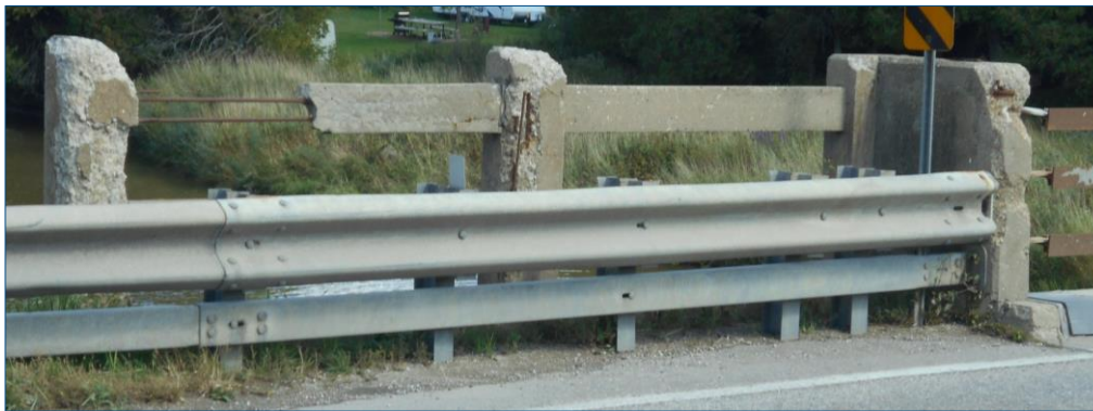
Concrete Railing with Spall and Exposed Rebar
