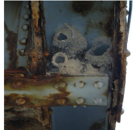
Cliff Swallow nests (>30) were documented on the underside of the Bridge in 2020
