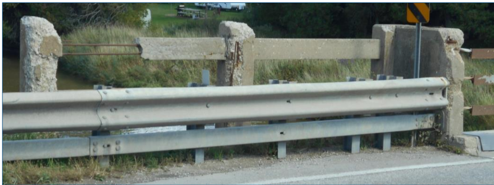
Concrete Railing with Spall and Exposed Rebar
