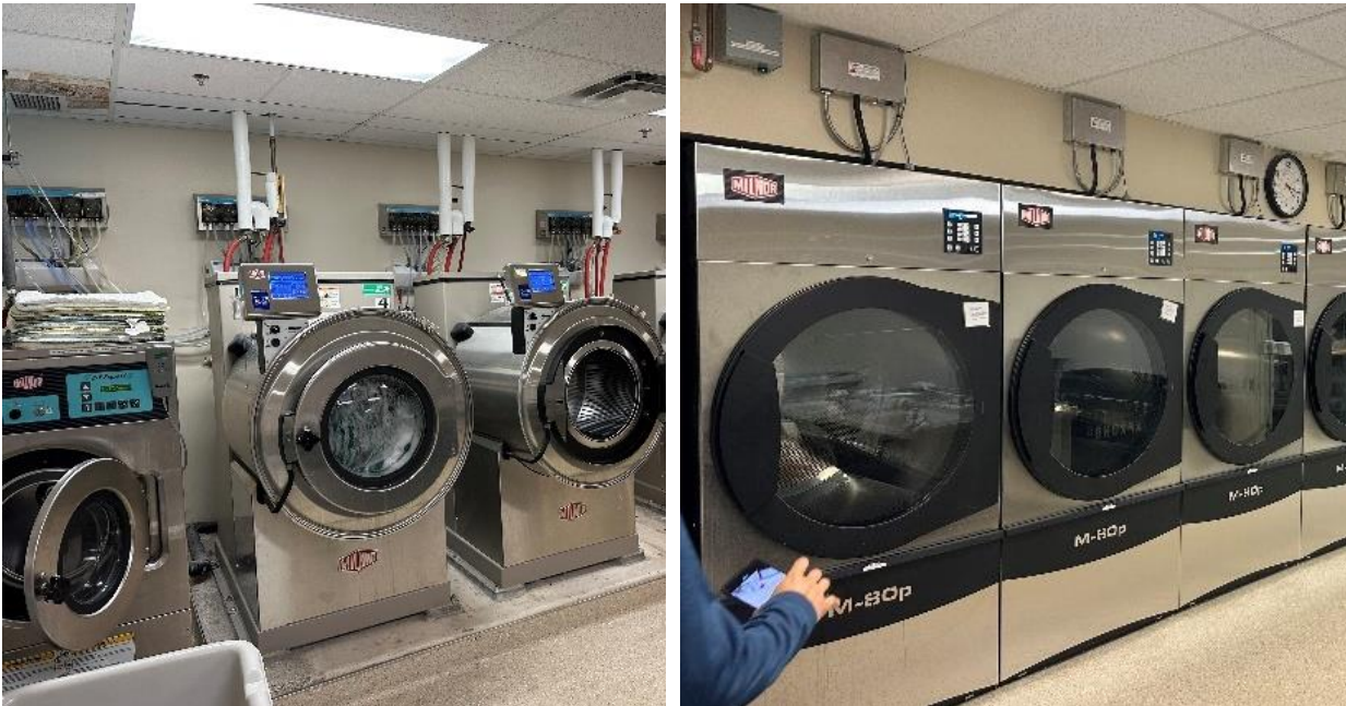
Figure 8: New washers (left); new dryers (right) at the Long-Term Care Facility
