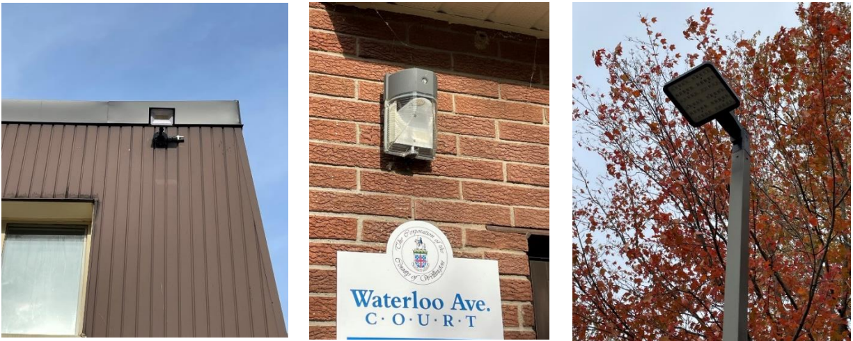
Figure 12: LED Exterior Lighting -387 Waterloo Court
