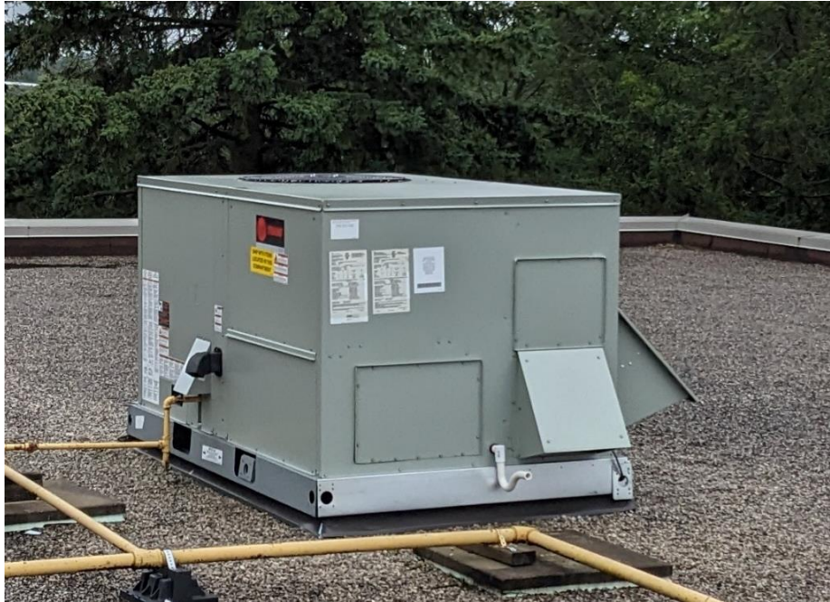
Figure 7: New roof top unit at Aboyne Library
