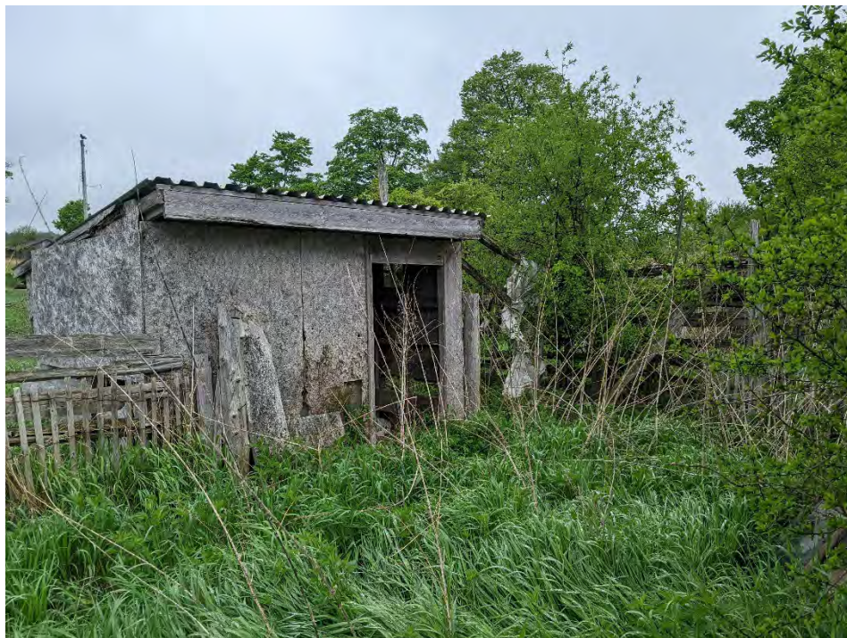
Photo 10 - View of the existing shed structure on- Site that may provide suitable habitat for bats. View facing southwest. June 22, 2022.
