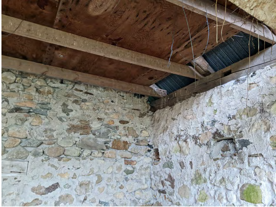
Photo 3 Photo of the barn structures that remains on Site. No bird nests evident.
