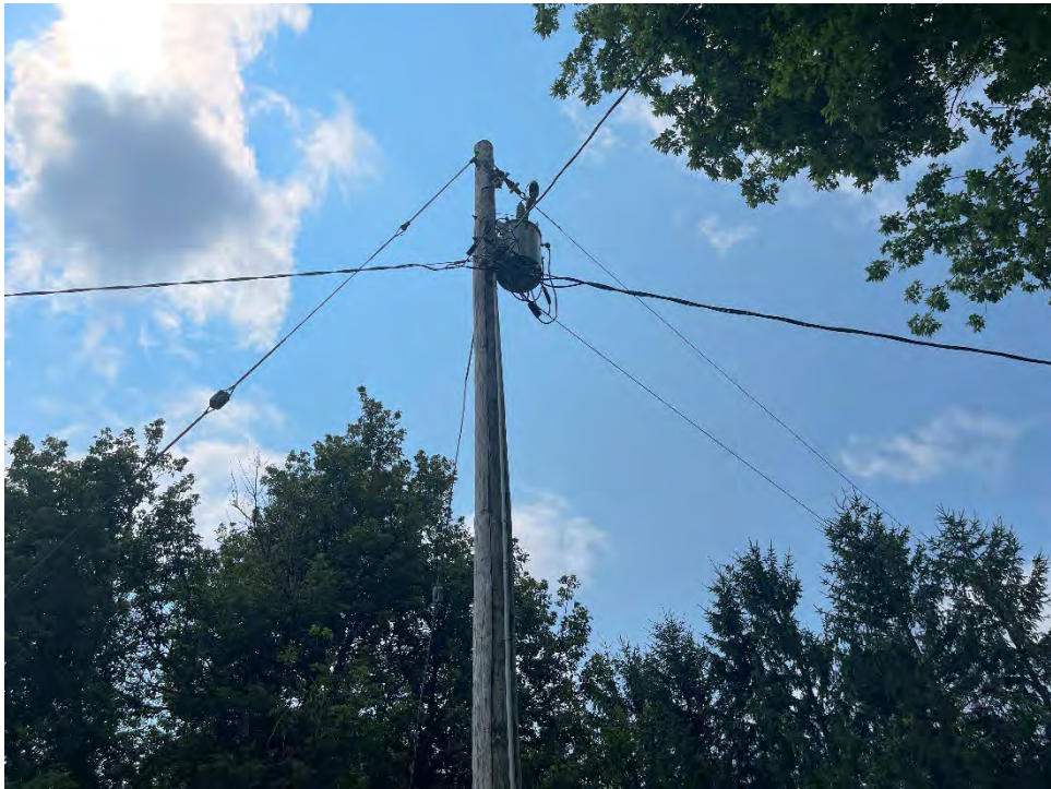
Photograph J10 – Pole-mounted transformer south of the maintenance garage. Facing southwest.
