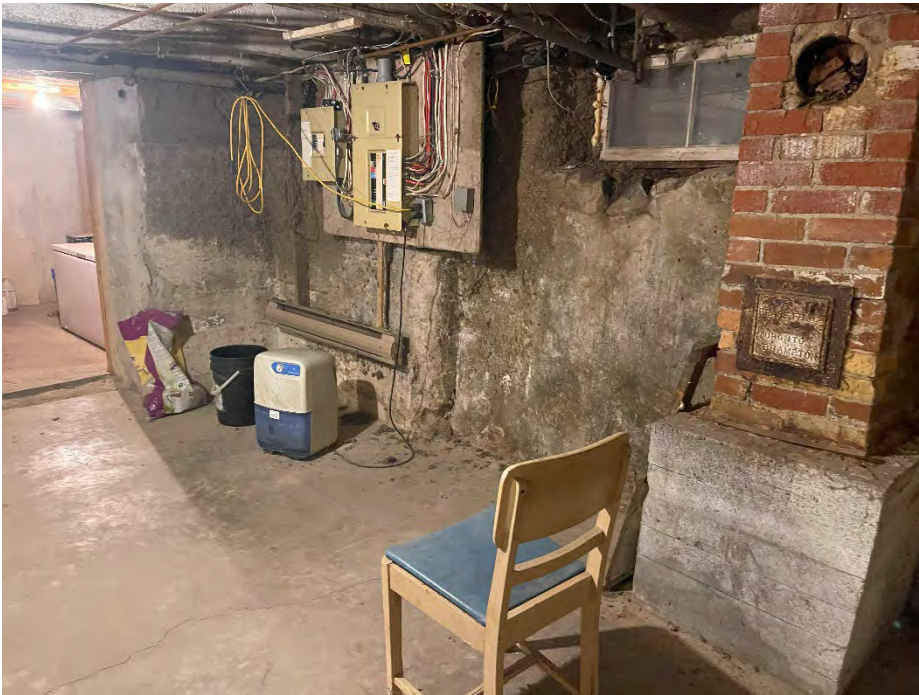
Photograph J6 – Basement of house, showing electrical panel and potential historical heating source. Looking southeast.
