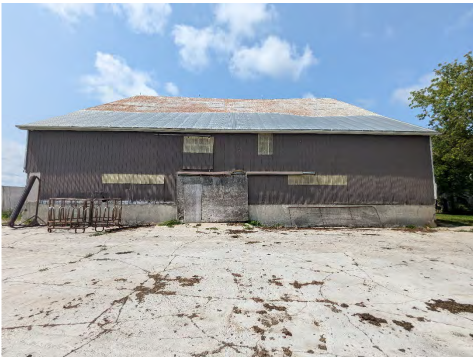
Photograph J4 – East side of barn and concrete pad used to dry out manure, looking west.
