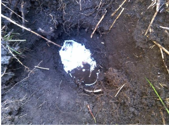
IMAGE 49 WATERLOGGED TEST PIT
