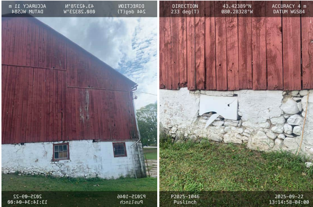
Photos 1 and 2: Exterior of the barn showing gaps that could serve as entry points for bats.
