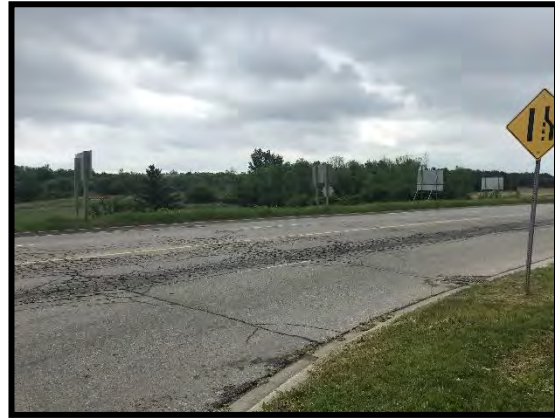
Image 2: Disturbed Lands – Roadway (May 31, 2018; Facing Southeast)
