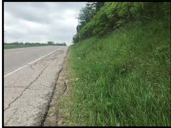
Image 12: Disturbed Lands – Roadway and Embankment (May 31, 2018; Facing South)
